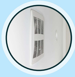
Whole House Ventilation System
